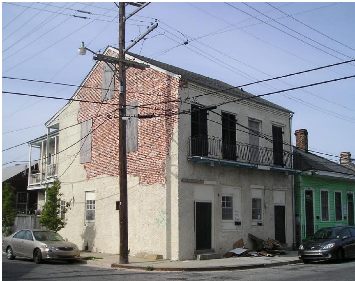
March 26, 2007 – Evidence of beginning of building stucco finish delamination cited by HDLC.
