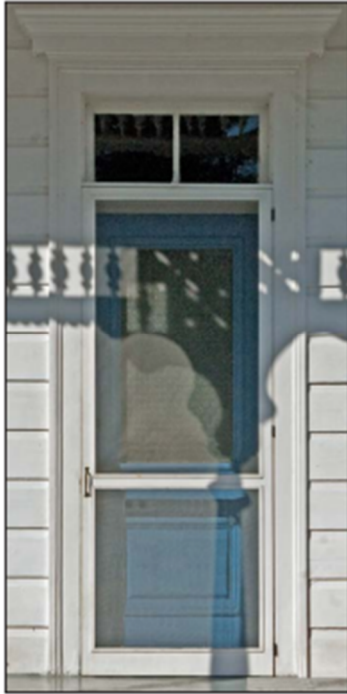
A screen door should be finished to match the historic door to provide protection from insects while minimizing the visual impact on the historic character.
